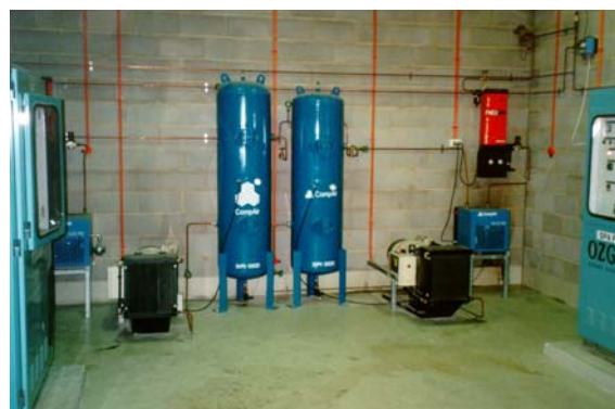
Figure 38 Air preparation plant for ozone generation
