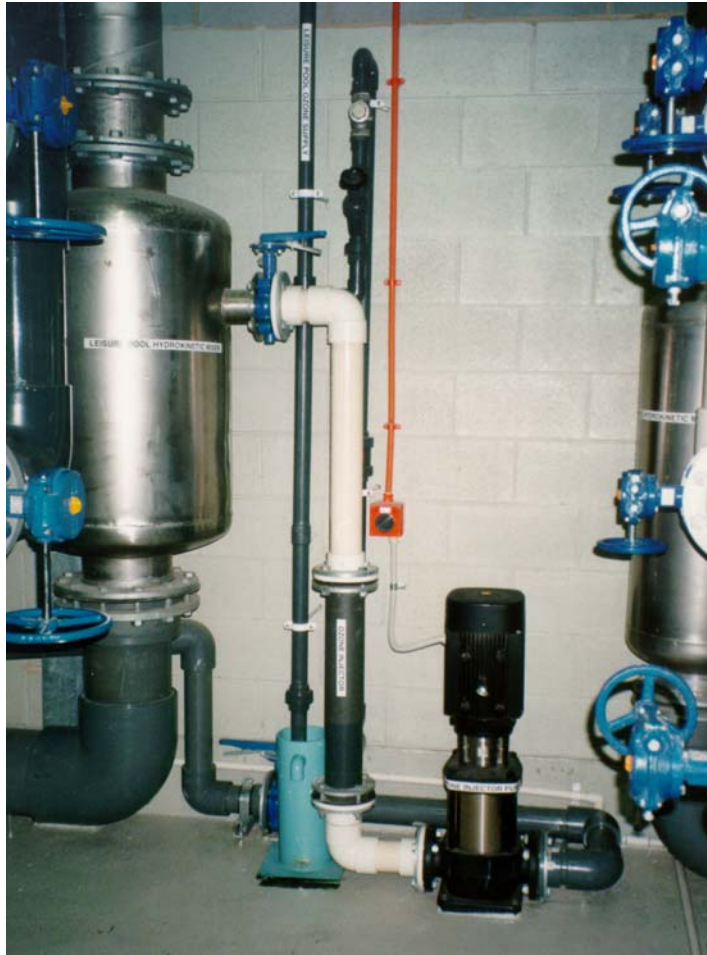
Figure 39-An ozone injection plant
